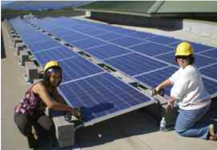
MEDB installed a new PV array on the rooftop of MEDB's Malcolm Center.
